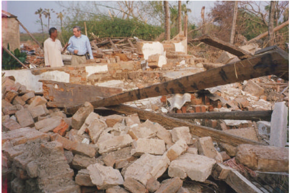
School Administrator Niranjan Biswal and Jay Wilson survey damage at the Tandikul Elementary School. Similar damage occurred to other essential facilities throughout the area.
